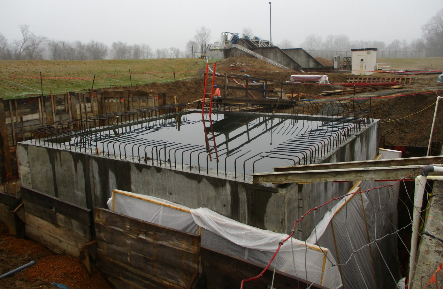
Stormwater Pump Station No. 1 - Photo 1
