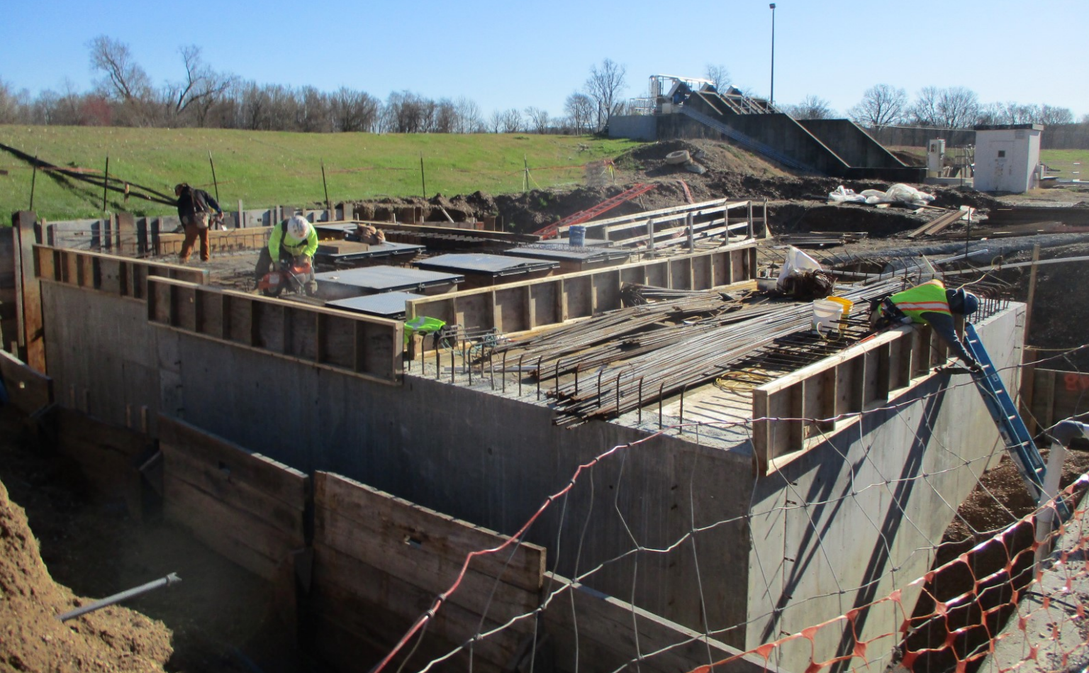
Stormwater Pump Station No. 1 - Photo 1
