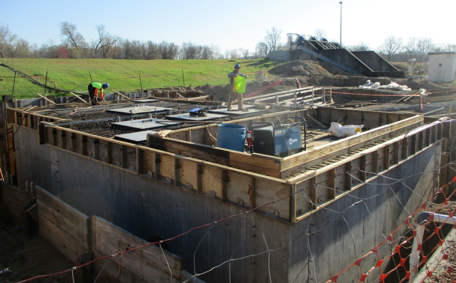
Stormwater Pump Station No. 1 - Photo 1
