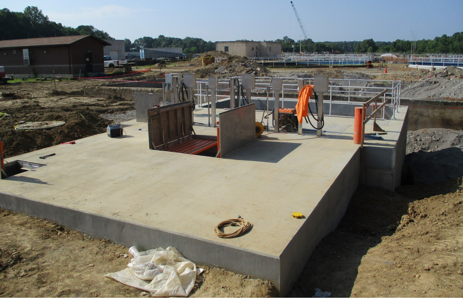
Stormwater Pump Station - Photo 3
