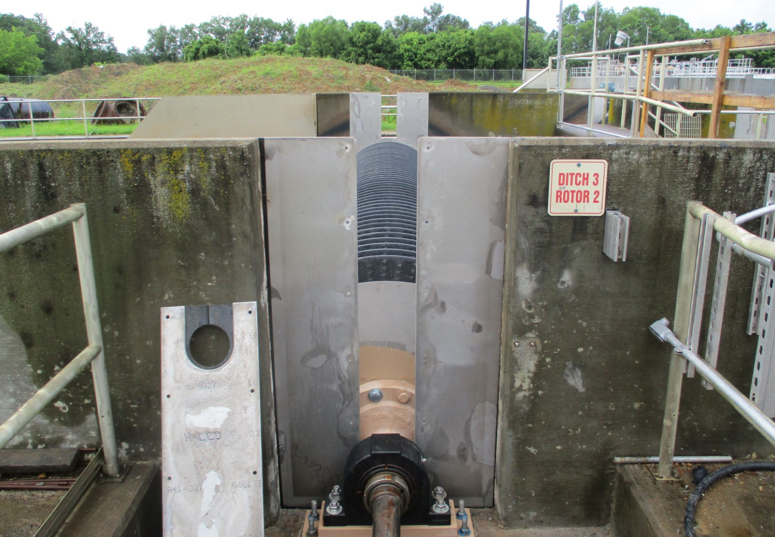
Oxidation Ditch No. 3 - Photo 1
