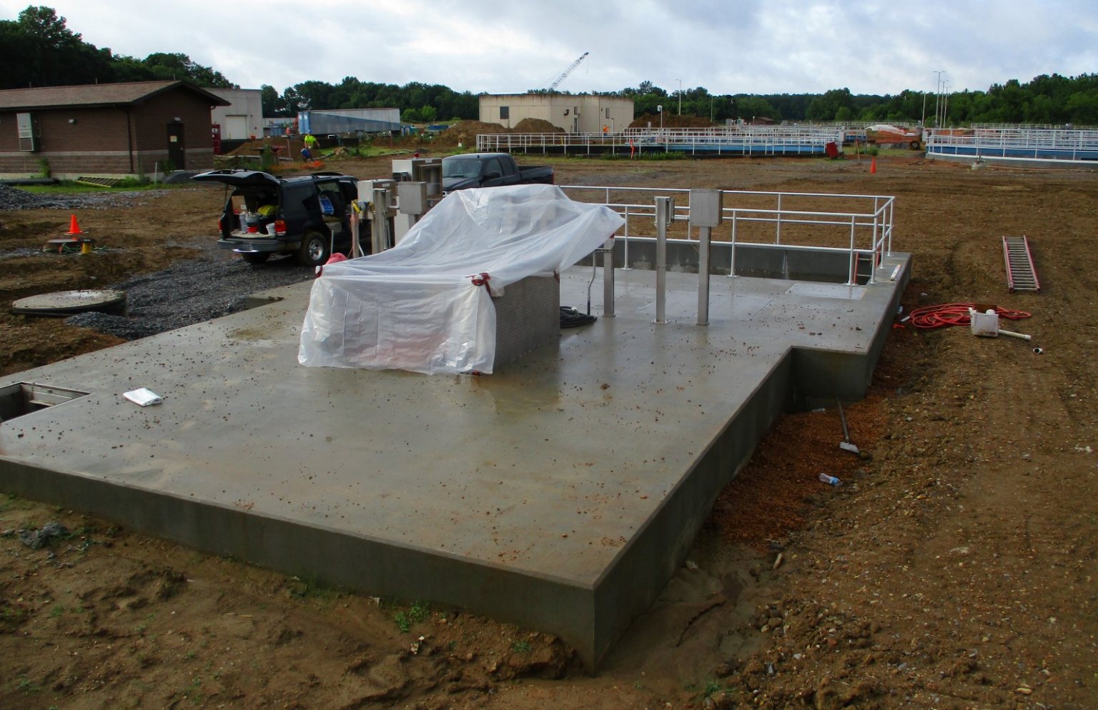
Stormwater Pump Station - Photo 3
