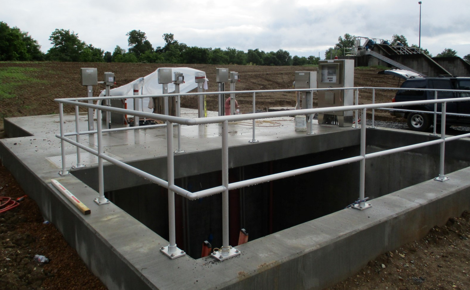
Stormwater Pump Station - Photo 1
