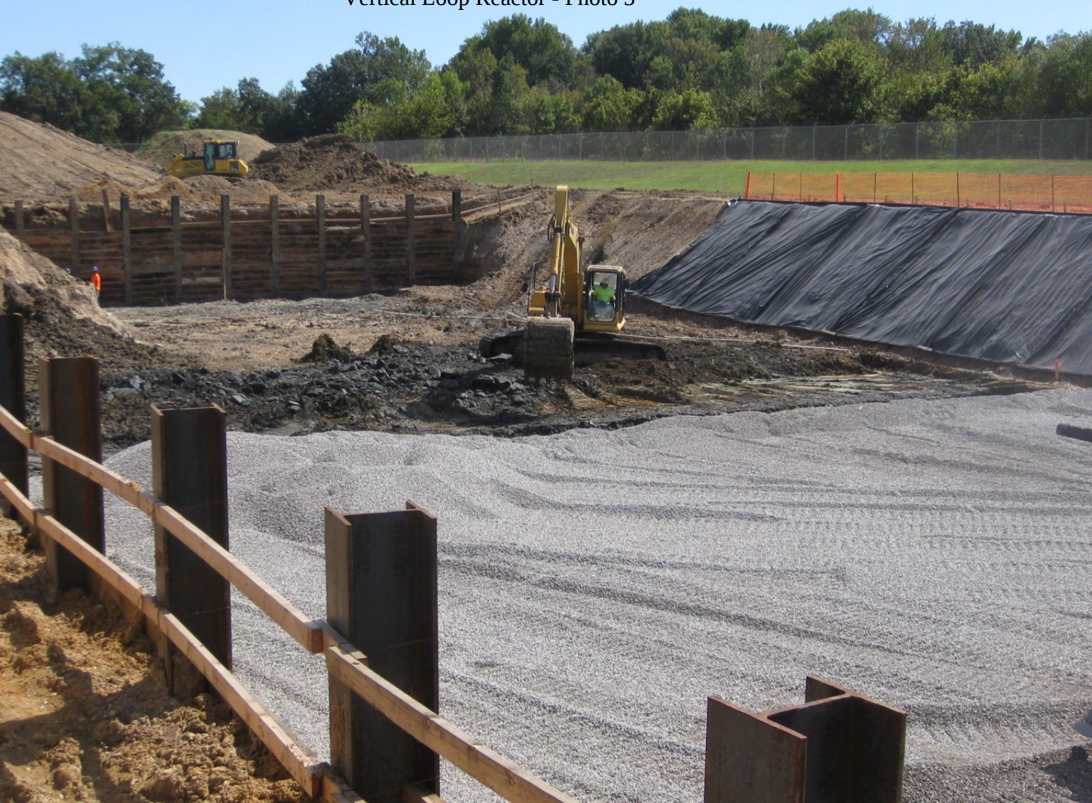
Vertical Loop Reactor - Photo 3
